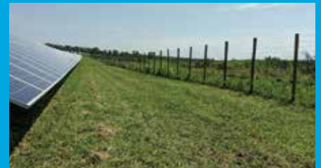
Array and Deer Fencing
